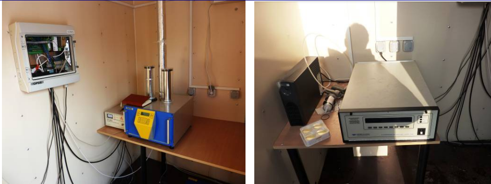
Kuklen Air Station-Monitoring Equipment
